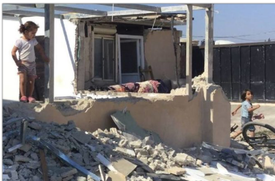
© OCHA OPT / Alternative Information Centre House Demolition, Jerusalem, Palestine, 2018
